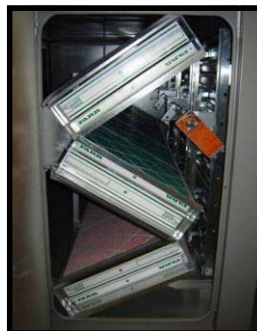
Filter and Damper Access
