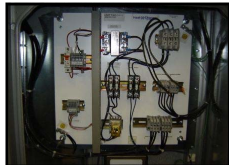
Single point power, Controls by others.
