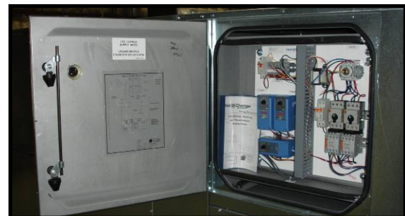
Energy Recovery and Airflow controls are configured in a simple panel.
