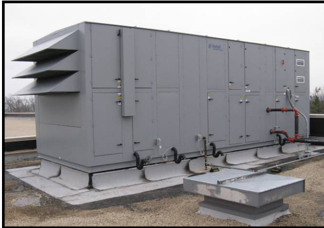
The Finished and Installed PXHS
