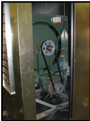
15hp Exhaust Air Blower
