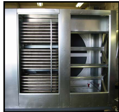
Supply Air (on left w/gas fired furnace) and Return Air (on right) through the heat wheel
