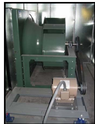
10 hp Return Blower
