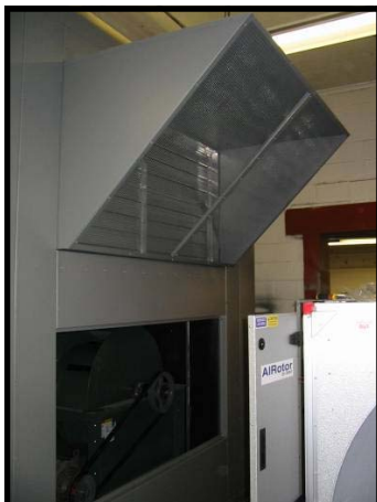
Exhaust Air Hood, Bird Screen, and Gravity Backdraft Damper
