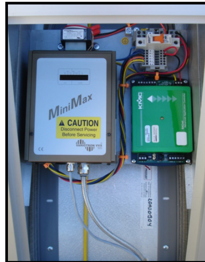
AIRotor DDC controller (right) alongside MiniMax multifunction heat wheel VFD (left)
