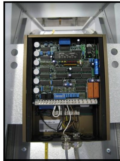
The AIRotor VFD, uncovered
