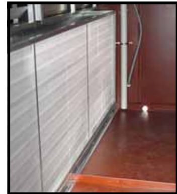
Cooling coil and Heresite-coated drain pans
