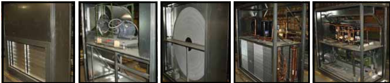
From left: The end section contains the OA damper; the next section contains the exhaust blower (top) and OA filter rack (bottom); the middle section houses the heat wheel; the next section contains the DX and Hot Gas Reheat coils (bottom) and two compressors (top); and the last section houses the twin supply blowers (bottom) and another two compressors (top).
